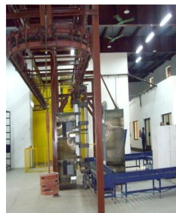
Gamma Radiation Facility at AERE
